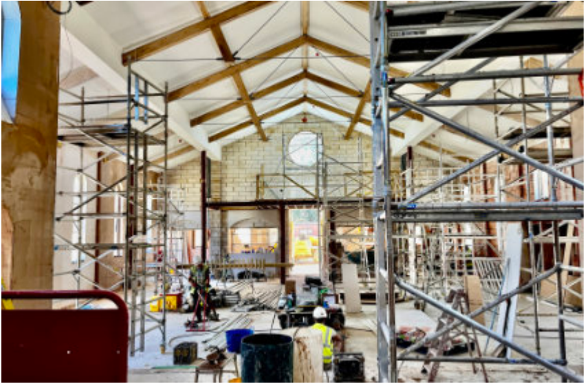
At St. Michael Archangel Chapel, work continues in a frantic push to finish before the end of October.
