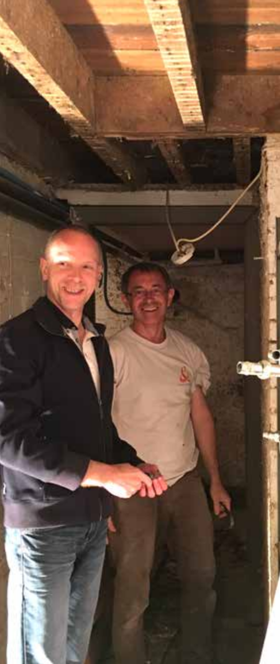
Two St. Michael's dads from Toulouse, France spent a week at the school to fix fireproof plasterboard to the ceiling of the cellar. May all their sins be expiated and may they be blessed for their generosity!
